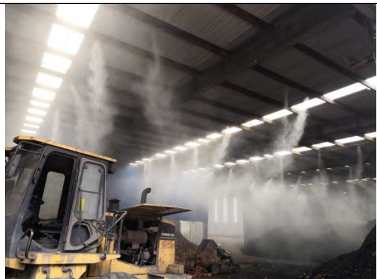
储库雾状喷淋
